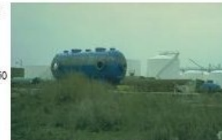
Above ground storage tanks
